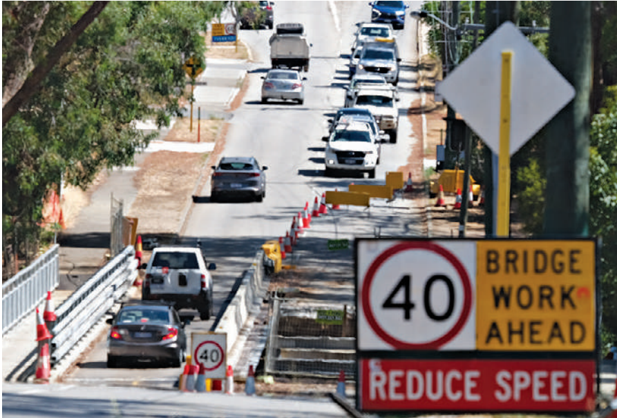
During construction, residents have experienced increased congestion and wait times. Picture: Andrew Williams
