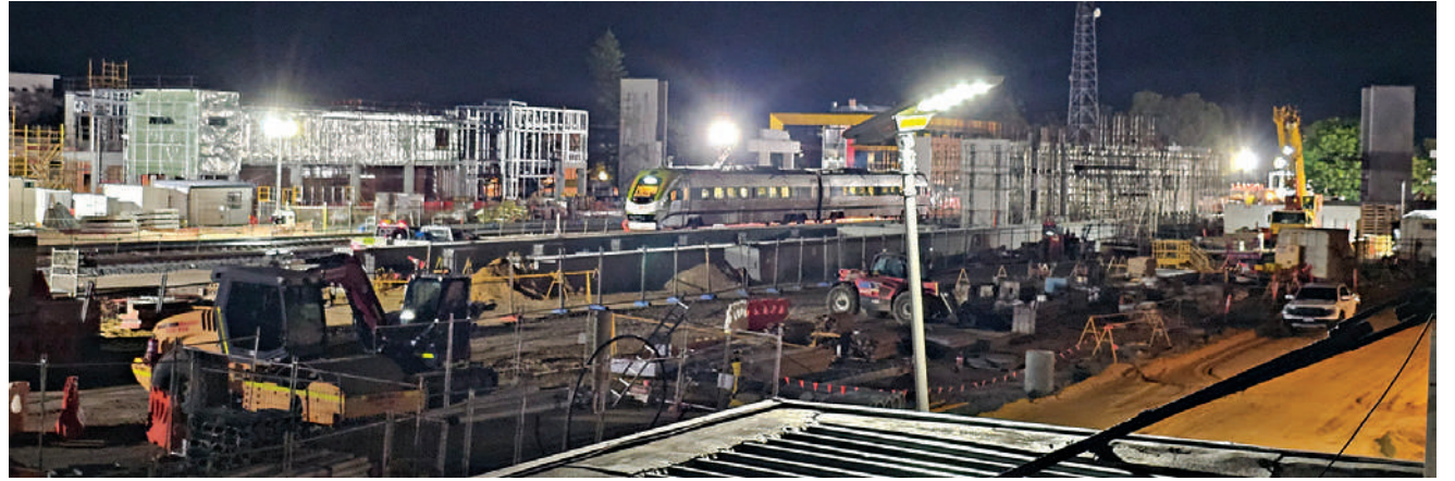
Railway Parade's out-of-hours worksite as seen from the Commercial Bar and Kitchen.
