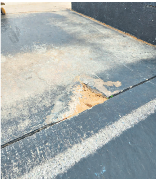
Cracks, worn surfaces and patchwork repairs at Ellenbrook skatepark have raised safety concerns among local riders.
