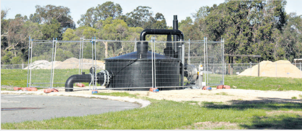
The odour control unit installed by Water Corporation along Millhouse Road. Picture: Camila Egusquiza Santa Cruz
